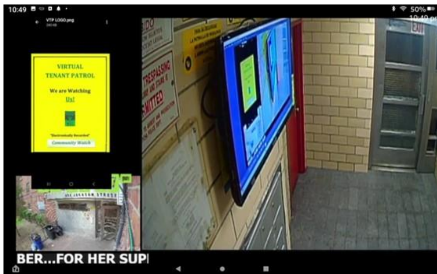
Resident Streaming Service Lobby
